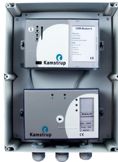
The inside of the data transceiver with GSM modem and radio concentrator.
